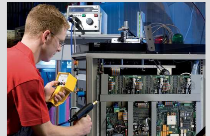
EN60204 test at a service cabinet
